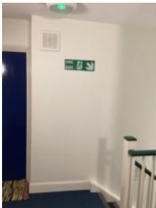
Escape route signage
