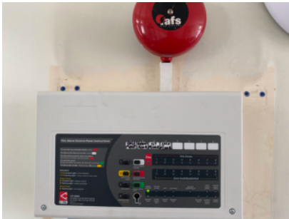
Recently installed fire alarm control panel
