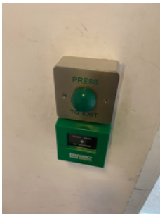
Electromagnetic entrance door release, with emergency door release device
