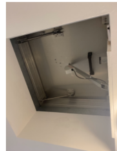
AOV provided at the head of the staircase.
