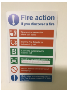
Incorrect fire action notice.
