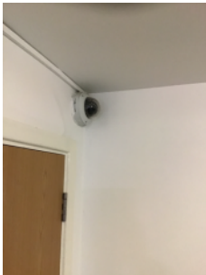
CCTV located in entrance hallway.
