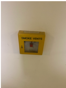
Smoke ventilation manual actuator is located in the staircase.
