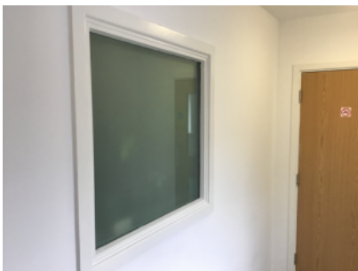
Flat glazing onto internal common corridors- no acids etching visible
