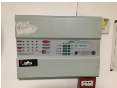
Fire alarm panel
