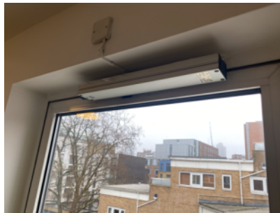
AOV (window) provided in the third floor corridor.
