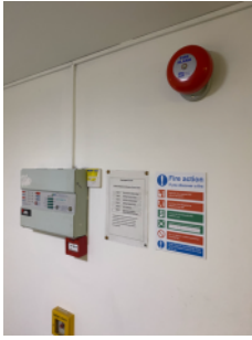
Photograph showing manual call point, sounder and fire alarm panel.
