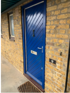
Example of flat entrance door without visible external self closing device
