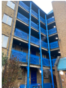
Photograph showing degraded insulating material around structural steels.
