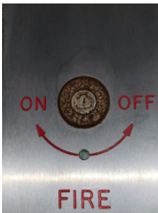
Rusted firefighters override switch to the lift.
