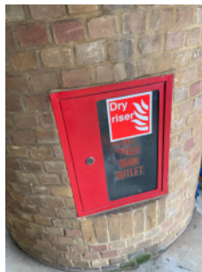
Dry rising main outlet
