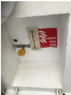
It was not possible to access the lift motor room
