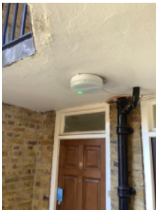
Maintained emergency lighting on common balconies
