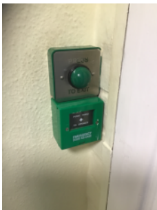
Main entrance door release, with emergency door release
