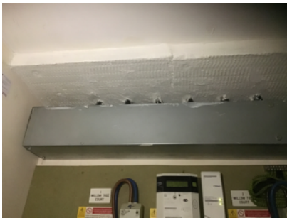
Good standard of fire stopping in the electrical cupboard
