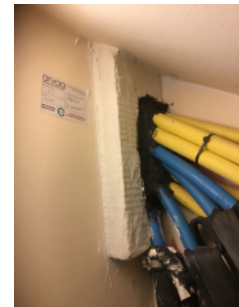
Good standard of fire stopping in the cleaners cupboard
