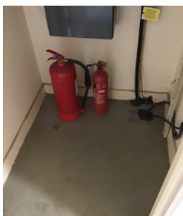
Extinguishers in electrical cupboard
