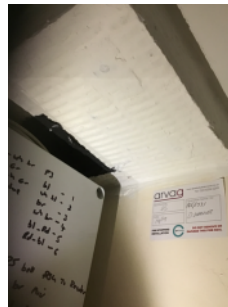
Good standard of fire stopping in the electrical cupboard
