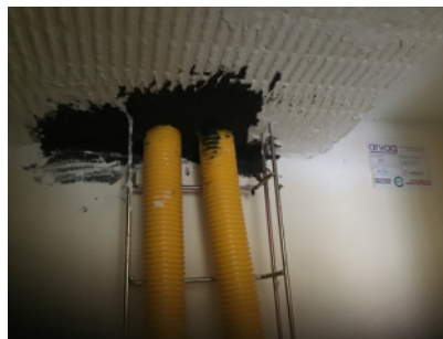
Good standard of fire stopping in riser cupboards.
