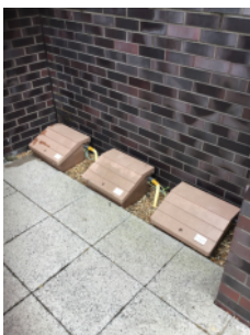
Gas meters located externally
