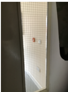
Georgian wired glazing in staircase door
