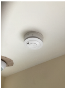
Part-6 detection in entrance hallway.
