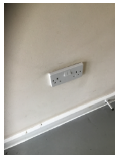
Electrical sockets provided in common parts of the building
